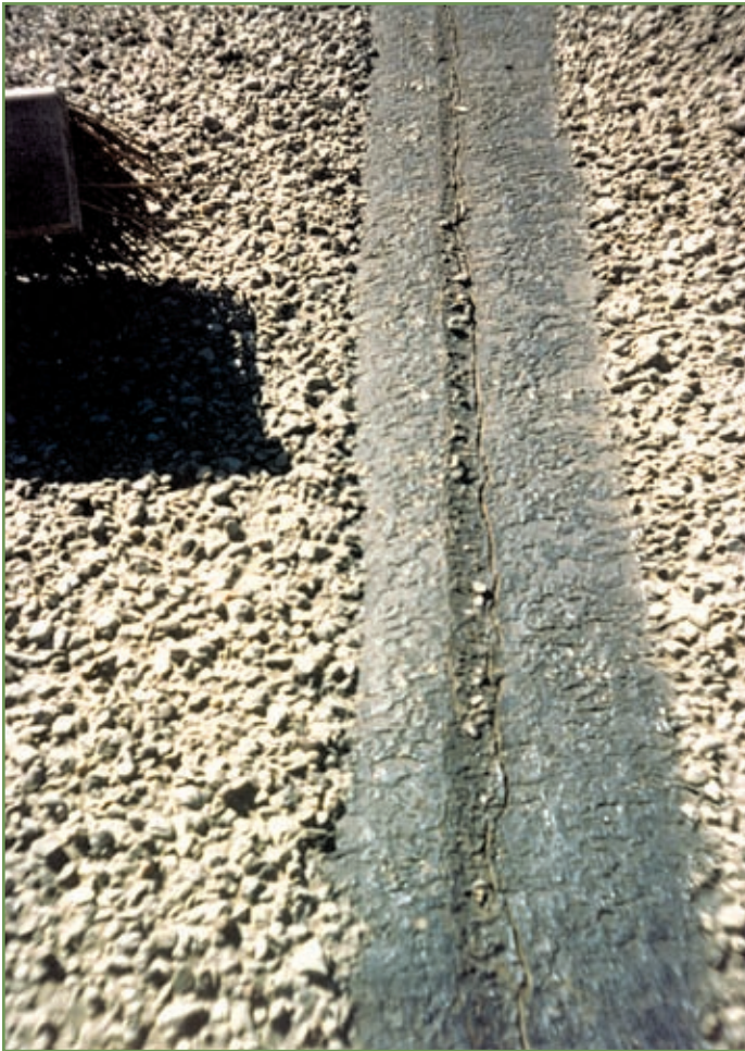
Exposed split at insulation joint.
