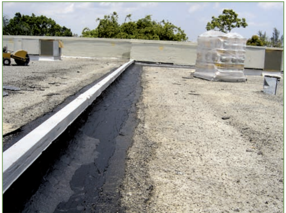
Note the wide spudded area at the base of this roof divider.
