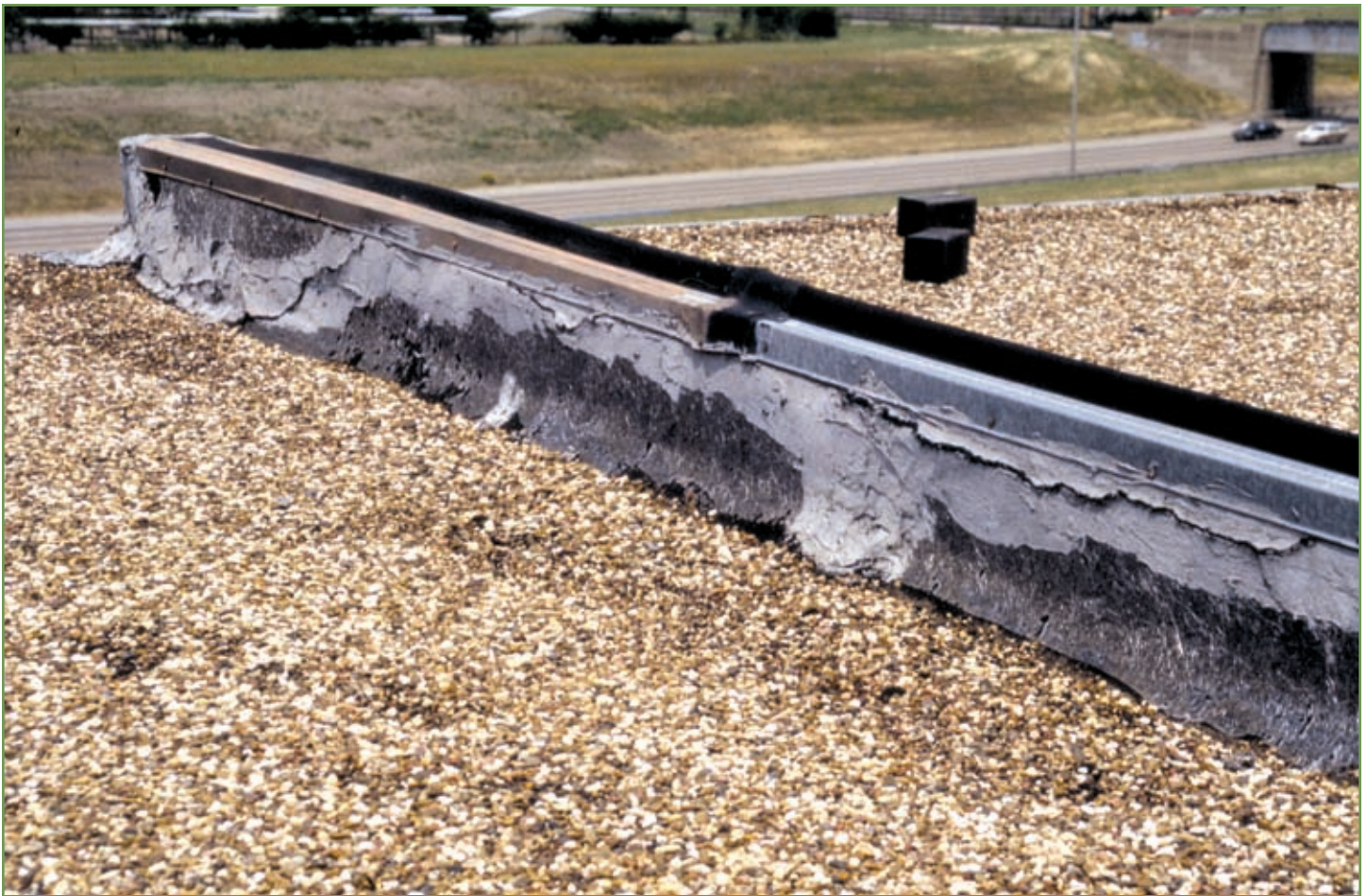
Splits at an expansion joint. Wall movement was not helped by the expansion-joint cover.
